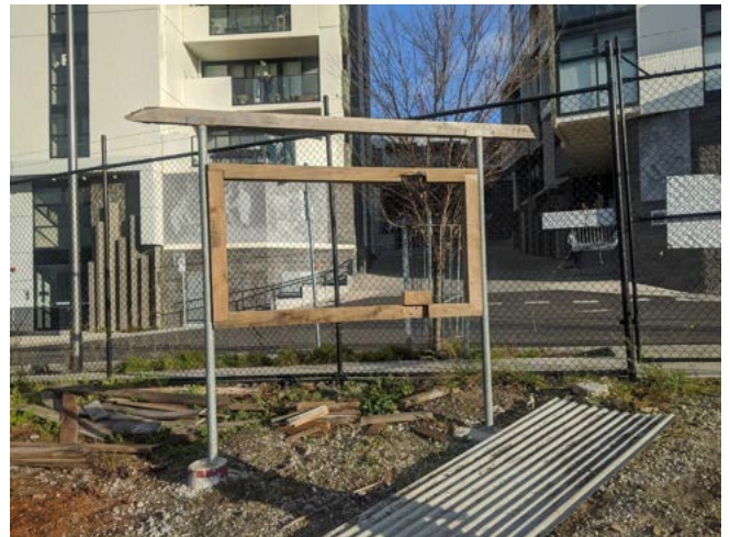
Photo 1: Construction has started on an informative sign next to the front gate
